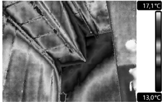
Figure 9. Thermogram of the upper corners with a visible temperature reduction in the corner
