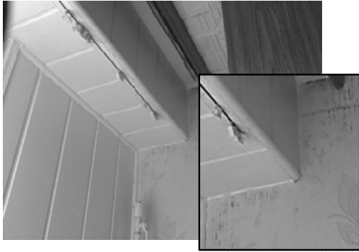
Figure 8. Photograph of upper corner connection gable wall – curtain wall with mold traces visible on the wallpaper
