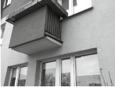
Figure 2. Balcony with the uninsulated plate
