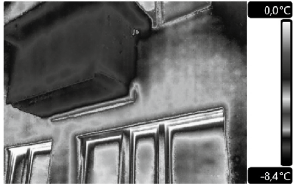
Figure 3. Thermogram of uninsulated balcony plate with visible thermal bridge
